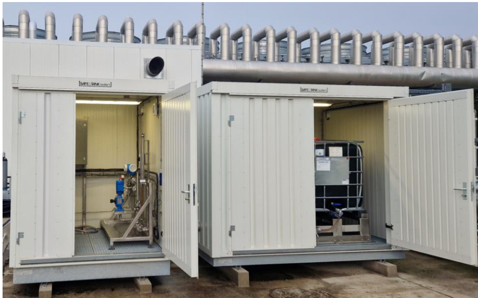
Inhibitor dosage station
