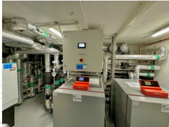
Figure 6: Boiler room view after implementation
