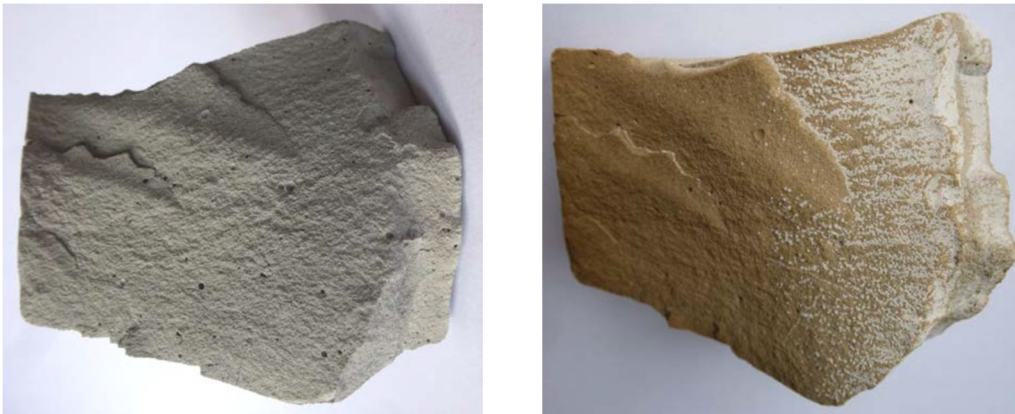
Fig. 7: Concrete sample before (left) and after experiment (right) V012. Brownish discoloration and white precipitates on the concrete is clearly visible [Anne Kaulisky].
