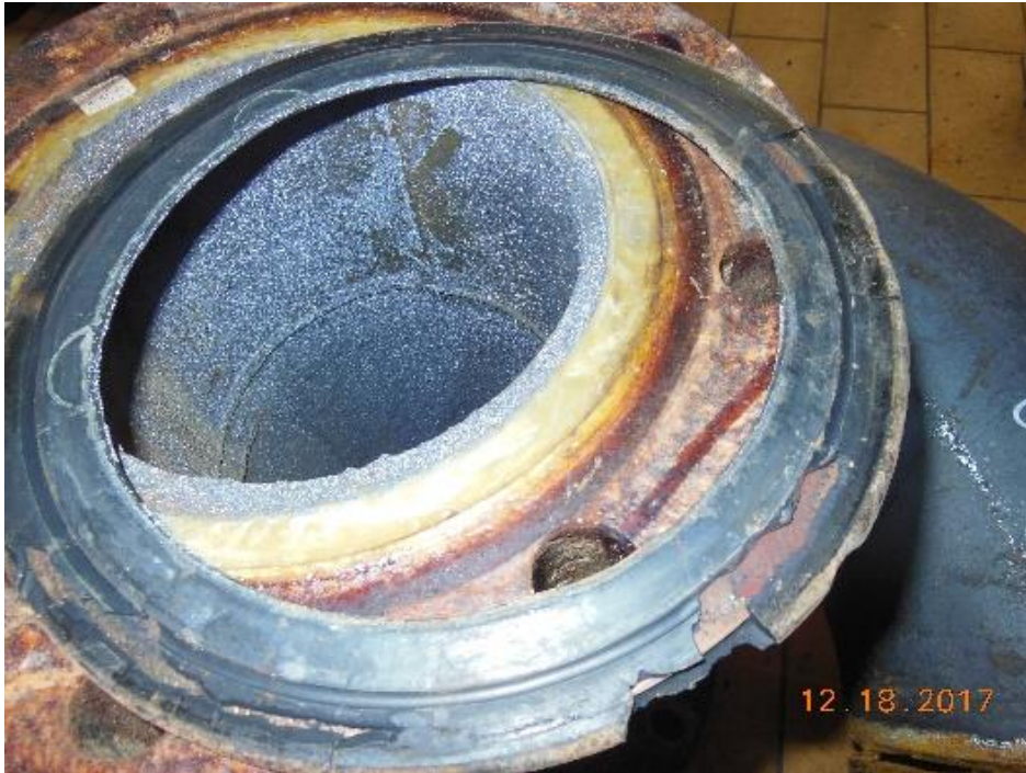
Destroyed gasket, EPDM (with scaling)
