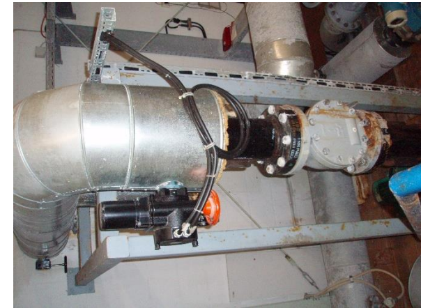
Typical leakage followed by corrosion
