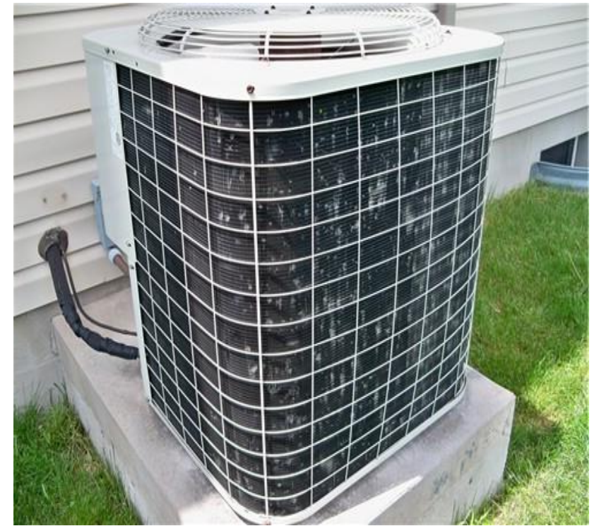
Remote Outside Condenser
